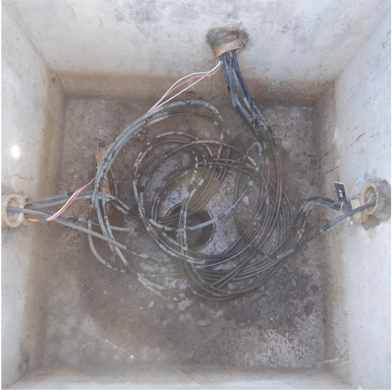
REIL 14 Hand Hole – RWY and REIL Wiring
