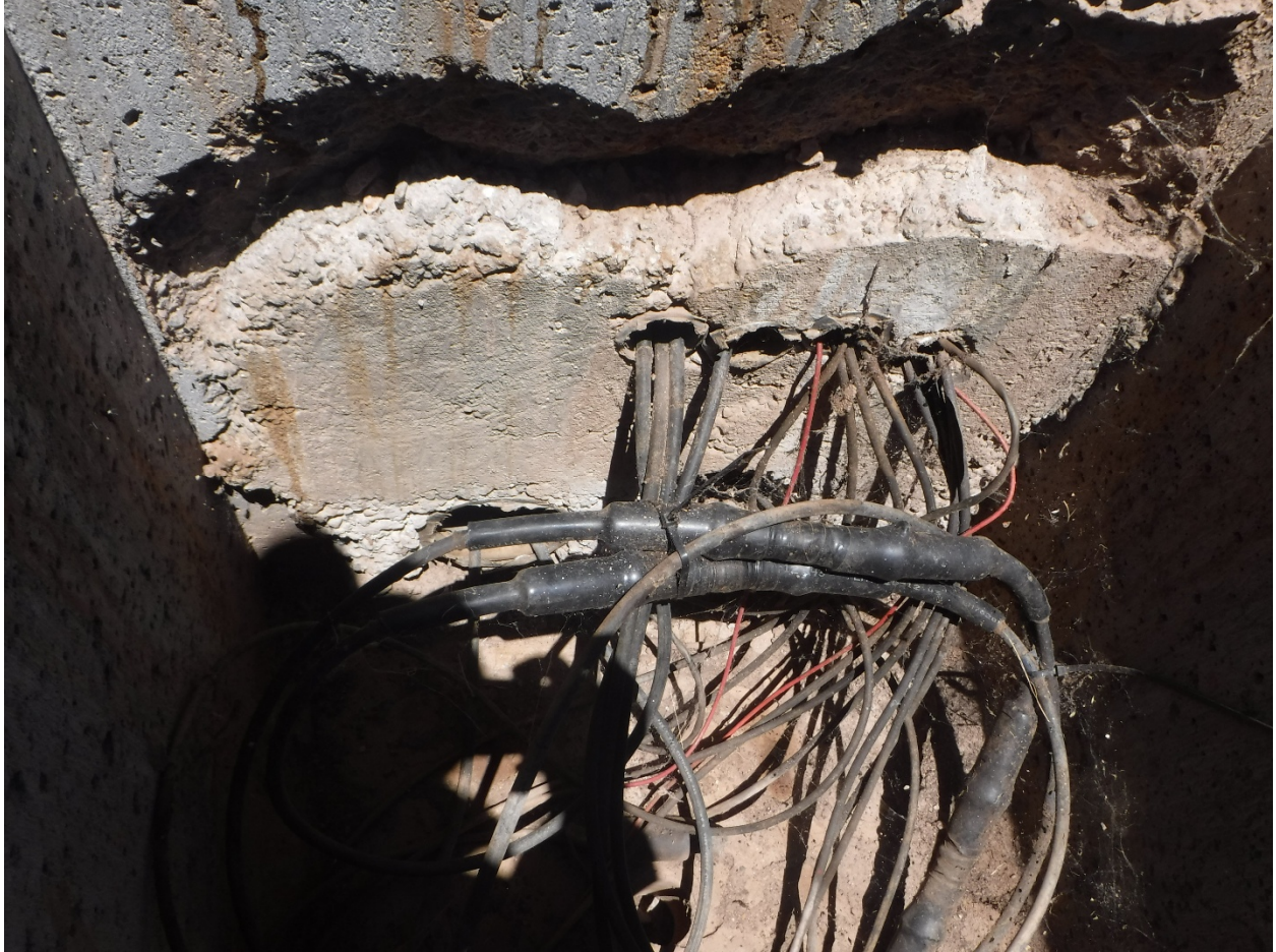
(REIL 32 HH at A1 and wiring)
