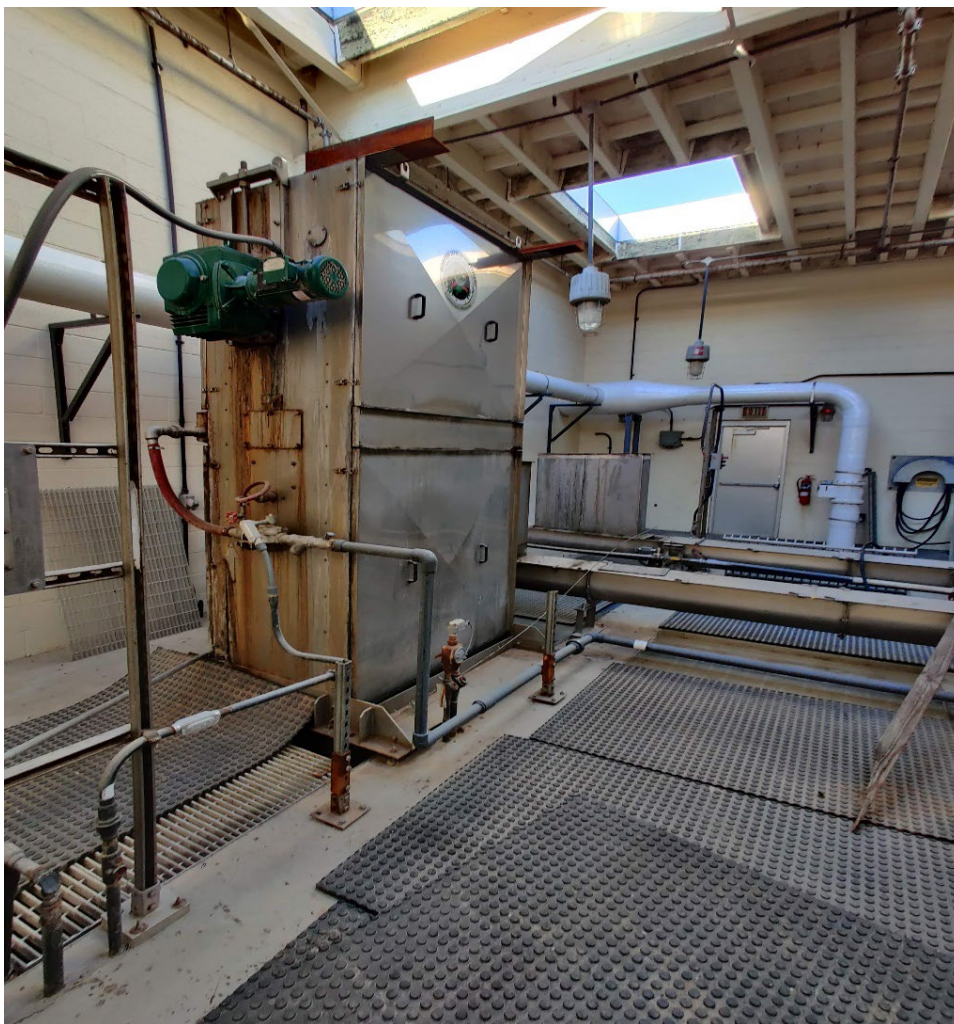
Figure E-2. Screen Enclosure Showing Signs of Corrosion
