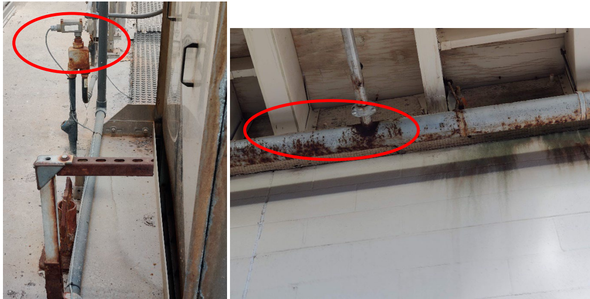
Figure E-3. Typical H 2 S Corrosion of the Electrical System and Fire Sprinklers
