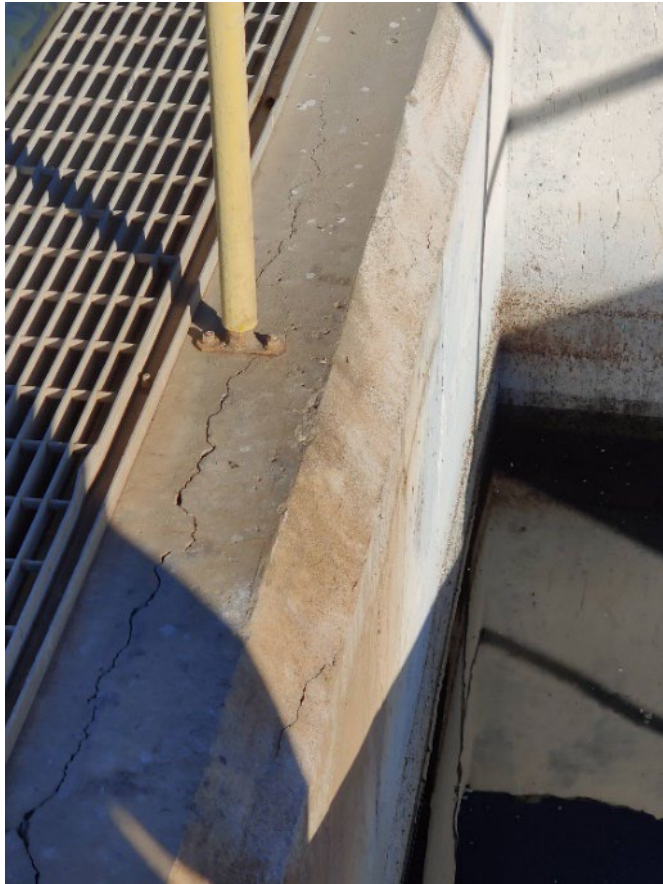
Figure 6-7. Cracks Observed in the Concrete Walls of the Sand Filter
