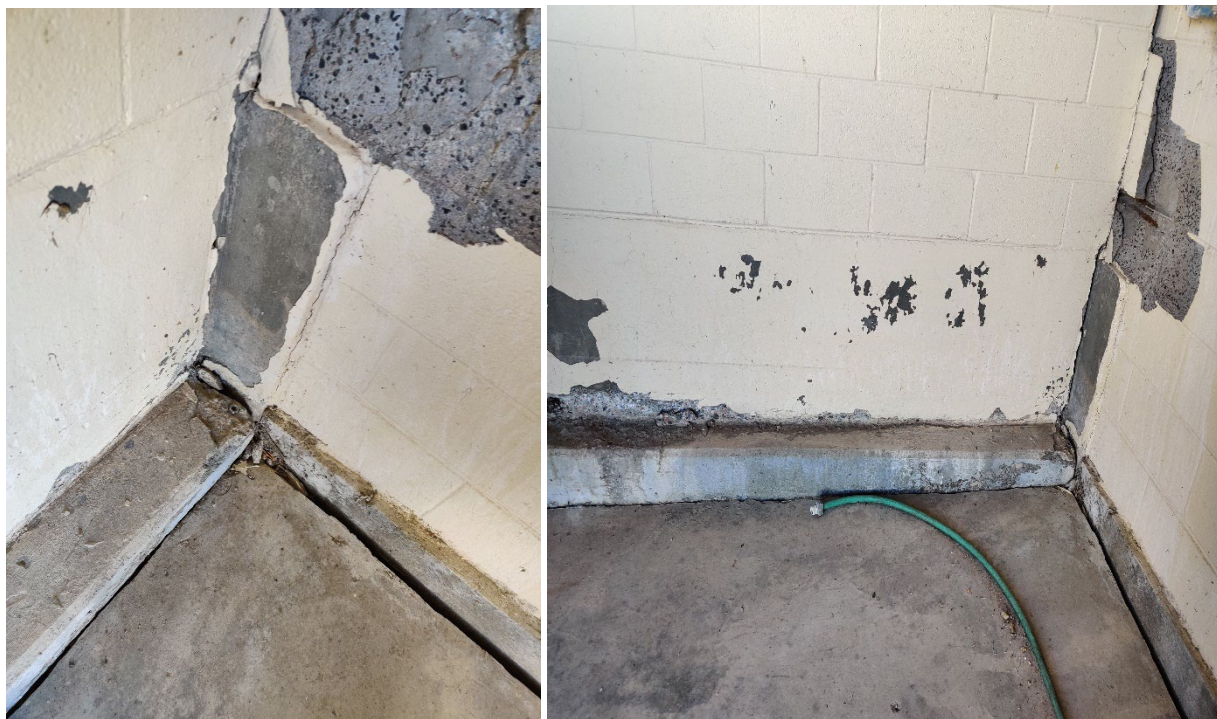
Figure C-2. Cracks Observed in the South Wall of the Headworks Building
